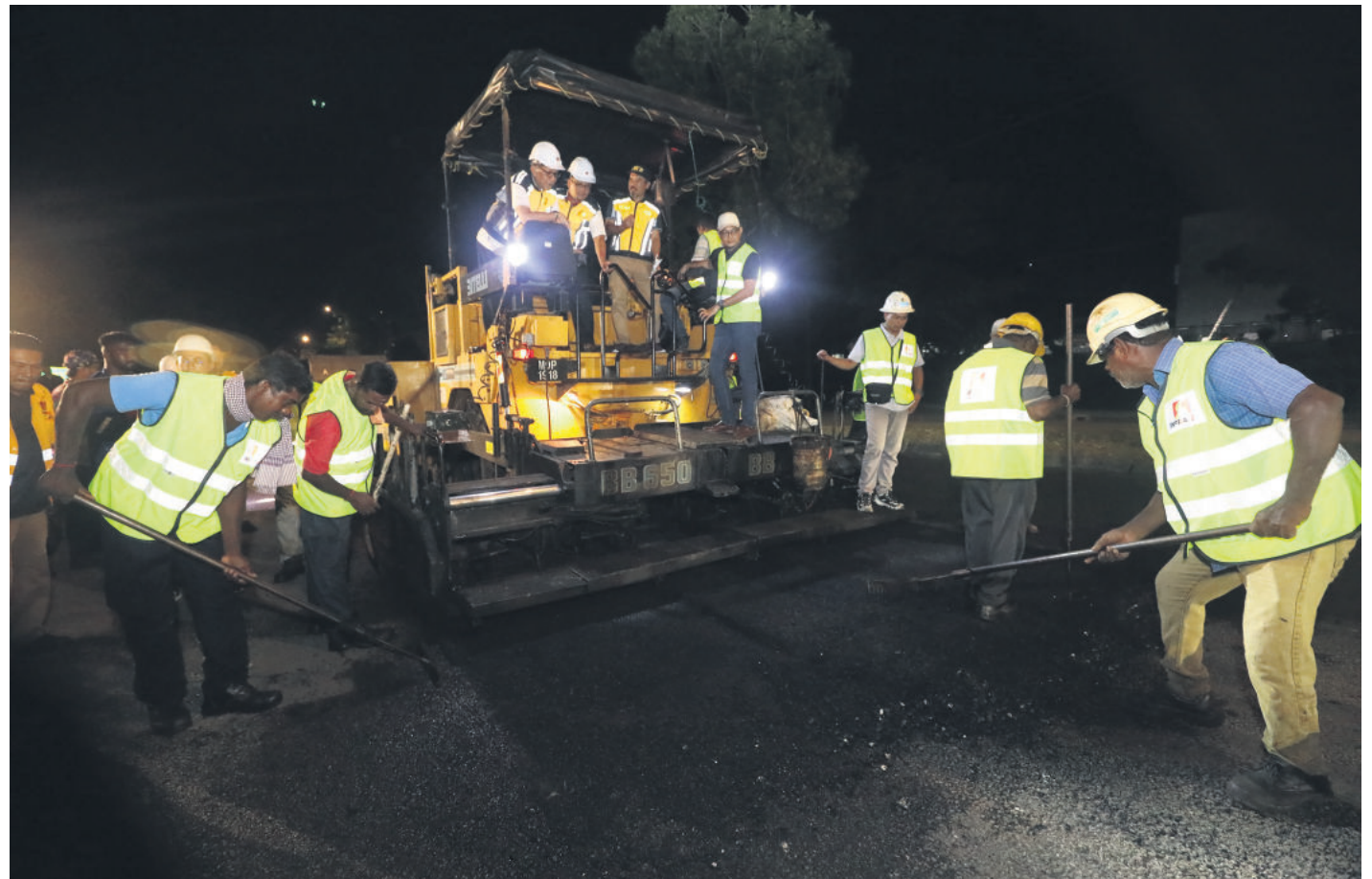
Roadworks being carried out at night at Jalan 22/1, Persiaran Jubli Perak in Shah Alam on June 1
